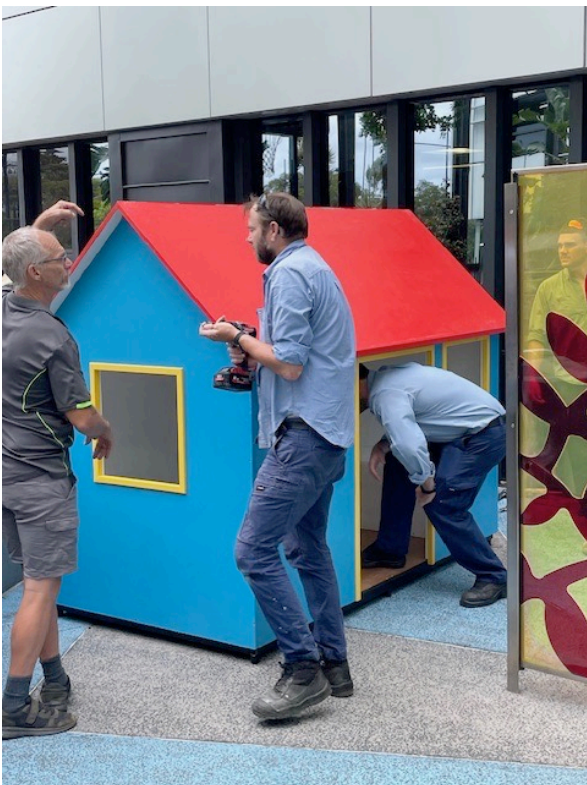
Erection of the cubby being undertaken by the hospital maintenance team under the watchful eye of Phil.
